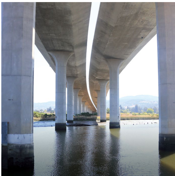
Caltrans repaired parts of the Maxwell Bridge over the Napa River after pieces of concrete cracked and fell during a 2014 temblor.
