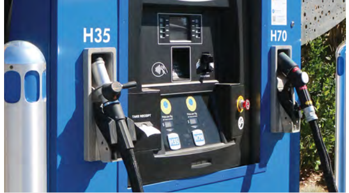
This hydrogen fuel station (there are 28 in the state), offers a half-pressure fill (H35, equivalent of a conventional half-tank), and a full fill (H70).
